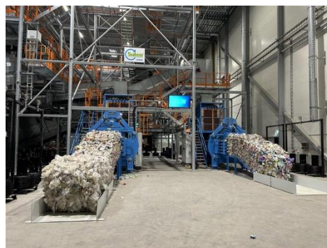
Finished Goods Baling
